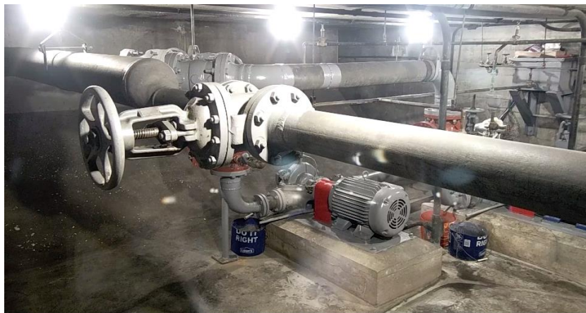
Figure 16 - Low Point Pump Station
