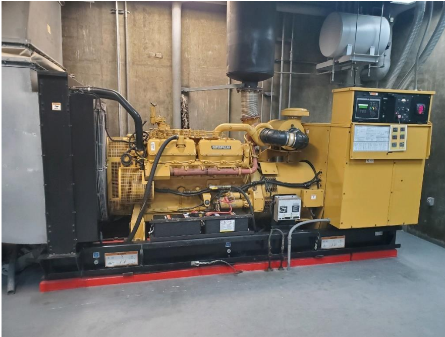
Figure 18 - Typical 500kW Emergency Backup Generator
