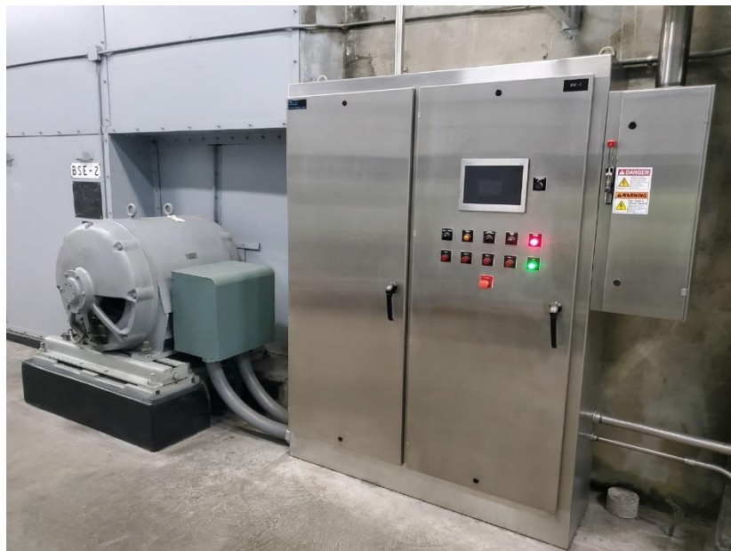
Figure 14 - Typical Fan MCC and Motor
