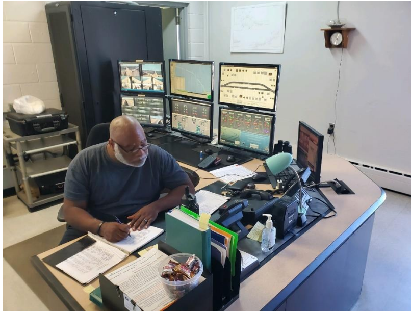
Figure 19 - Typical Control Room
