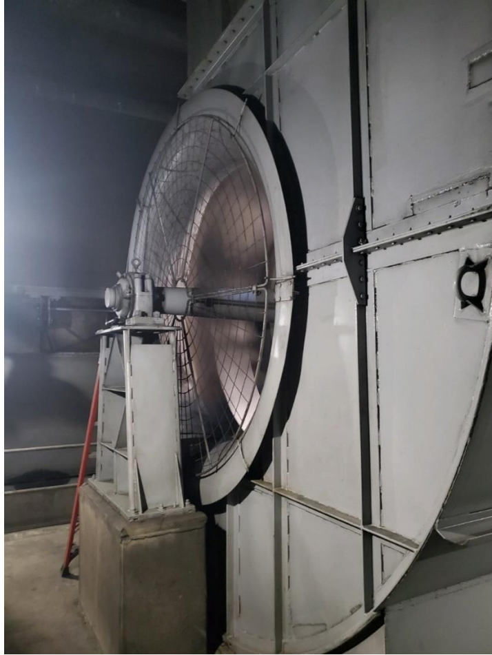
Figure 13 - Typical Exhaust Fan Room
