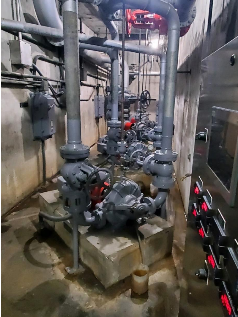
Figure 15 - Typical Pump Room
