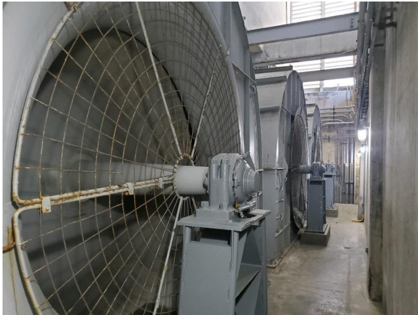
Figure 12 - Typical Intake Fan Room
