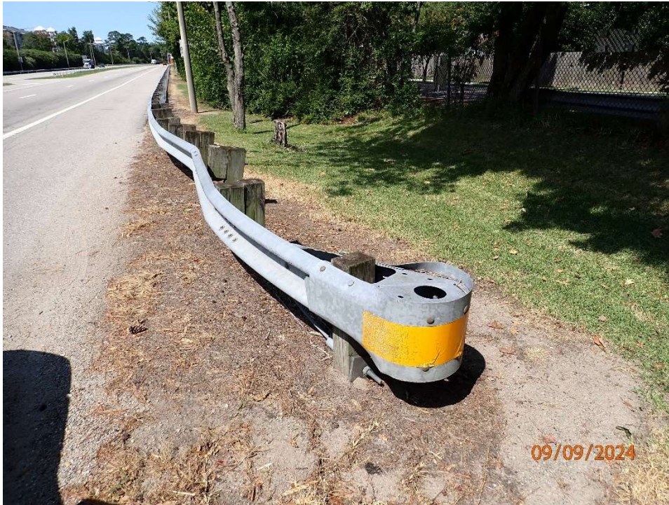
Photo 98: Approach Roadway (South); impact damage to guardrail pushed back up to 1' back (non CBBT property)
