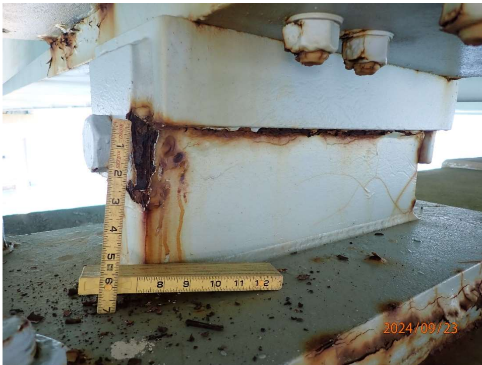
Photo 43: NCB-SB5 Bearings – Typical Peeling Paint with Surface Corrosion at Bearings (Looking Southeast)
