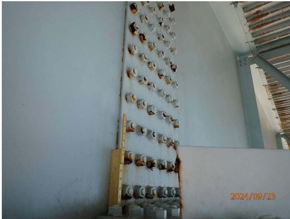
Photo 42: Superstructure – Blistering paint and corrosion on bolted connections.
