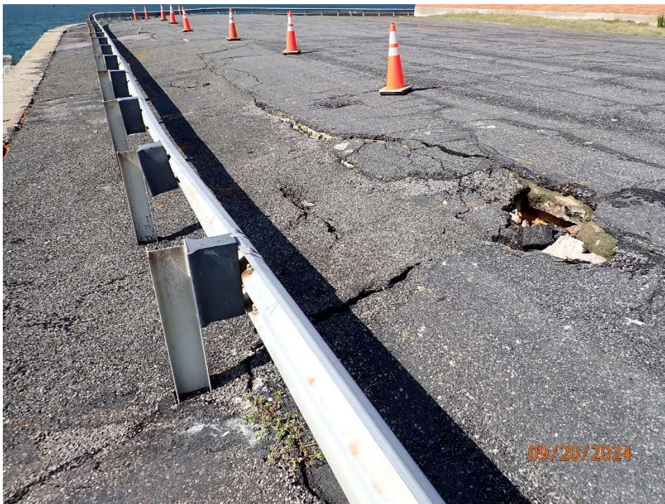
Photo 113: Portal Island 4 Splash Wall; Repair to previous sinkhole with urethane material. Sinkhole is still present in roadway with void under asphalt at time of inspection. The District noted in December 2024 that repair was made to this location.
