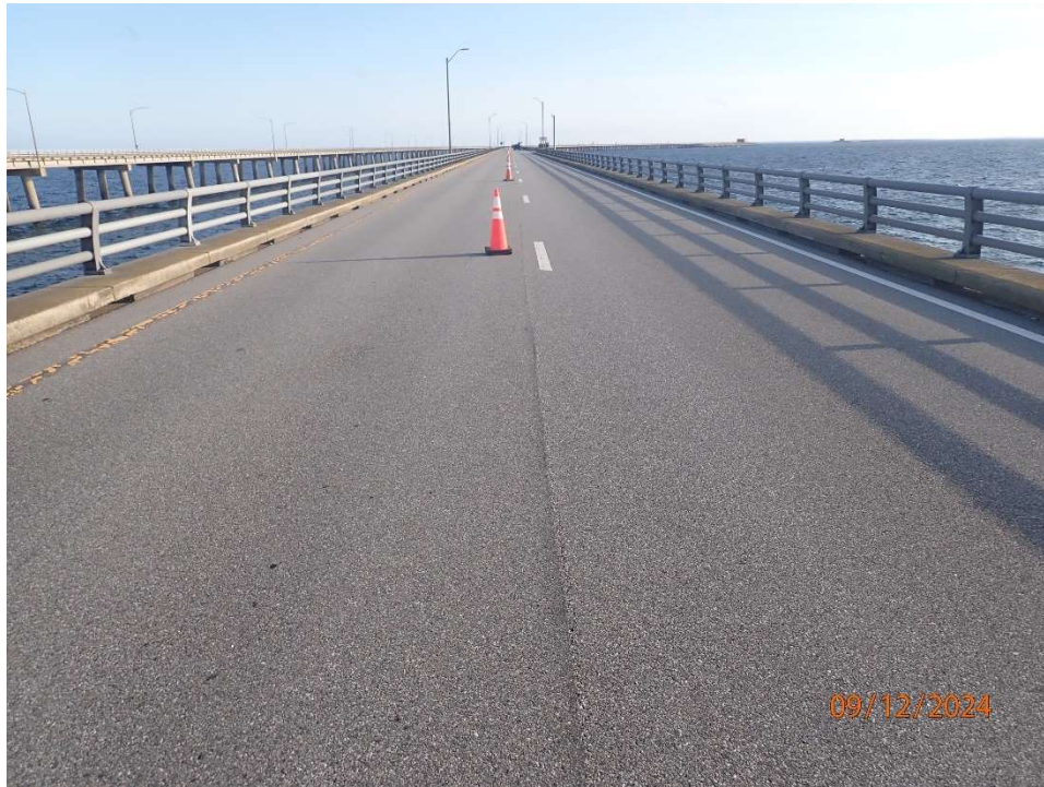
Photo 13: BNB160 – Asphalt wearing surface in good condition with pavement marking peeled and cracked.
