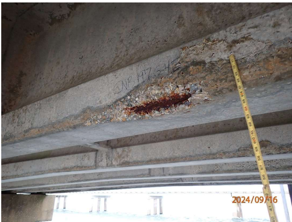
Photo 31: CNB197 Beam 4, Bay 3 1/3 span – spall 30" L x 5" H x 5" under x 1-1/2" deep with exposed prestressing strands with L1 having 10% loss of section.
