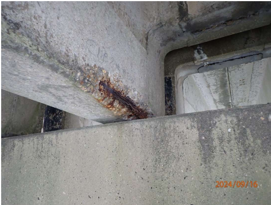
Photo 30: CNB206 Bent 207 Beam 5, Bay 4 – spall 30" L x 6" H x 5" under x 1" deep with exposed reinforcement with up to 100% section loss.
