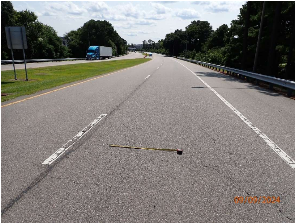
Photo 96: Approach Roadway (South) near Trestle ASB; Asphalt with alligator cracking up to ¼" wide throughout.
