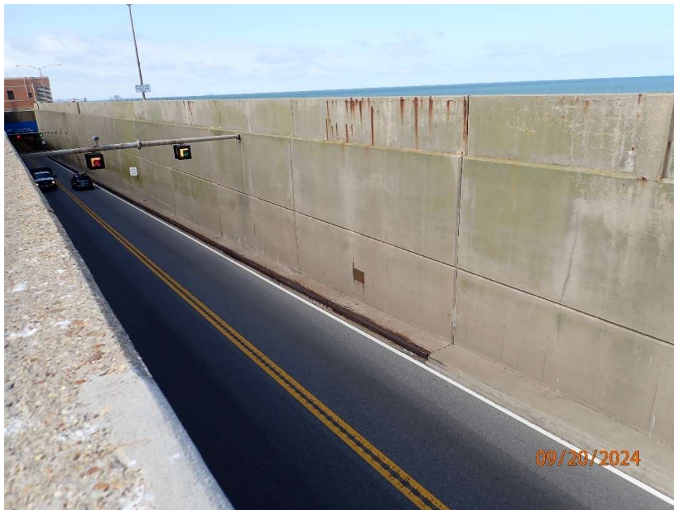
Photo 111: Portal Island 4: Open Approach Roadway and Walls; typical condition .
