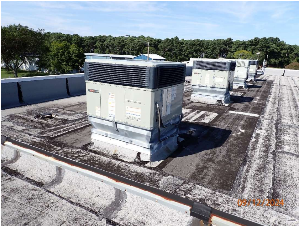
Photo 128: North Toll Plaza, Toll Booth and Canopy with roof in good condition.
