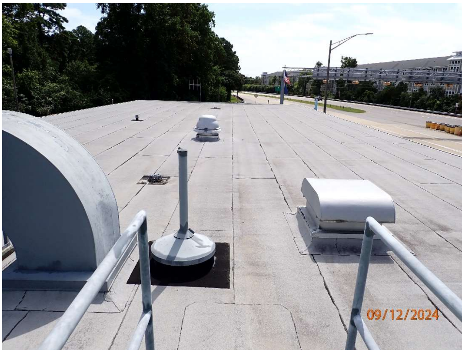
Photo 119: South Toll Plaza; Toll Office Building Roof in good condition with no notable defects.
