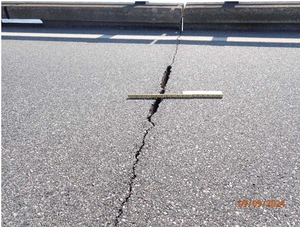
Photo 3: ANB183 Open Expansion Joint – spall 2' L x 1" w over expansion joint with \frac{1}{4} " transverse crack full width (typical).
