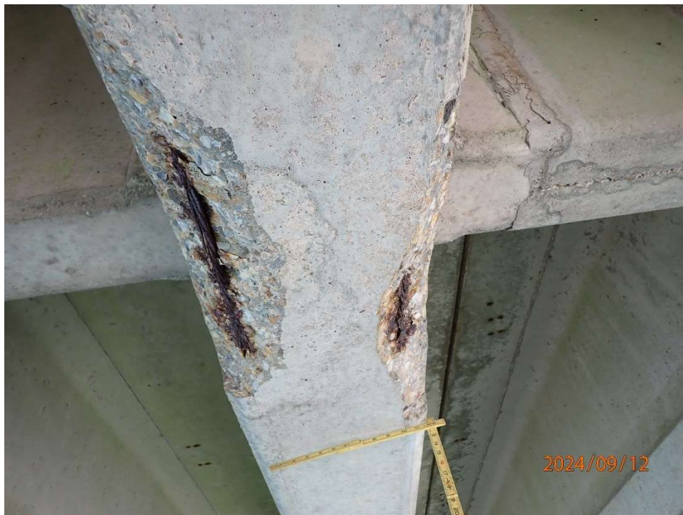
Photo 18: BNB192 Beam 5, Bay 5 at 1/3 span – spall 28" L x 4" H x 5" Under x 1-1/2" D with 1 exposed prestressed strand with 90% section loss and Bay 4 – spall 24" L x 4" H x 3-1/2" Under x 1-1/2" D with 1 exposed prestressed strand with 50% section loss.
