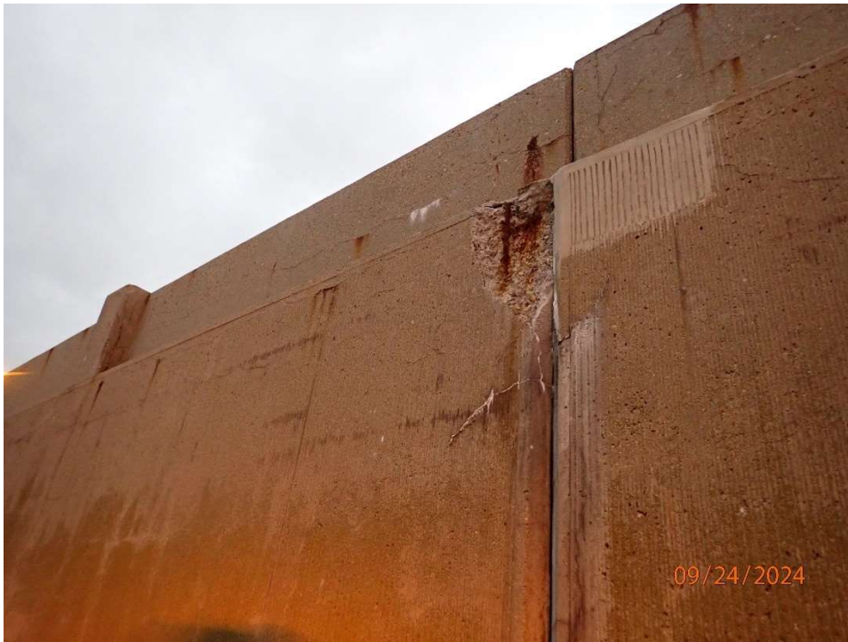
Photo 104: Portal Island 3 Open Approach Wall (east face); spall with exposed reinforcement with up to 100% section loss. Spalls noted at isolated locations and typically in the top 8' of wall.
