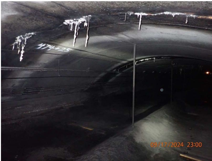
Photo 90: Exhaust Air Duct – General View of Random Transverse Cracking with Significant Efflorescence and Leakage in the Tunnel Liner (Looking West)
