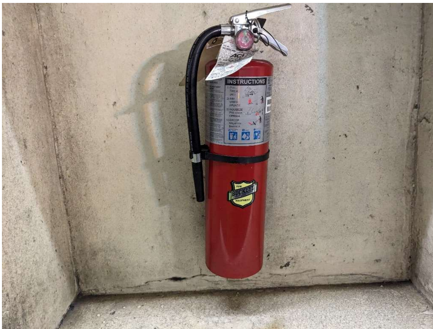
Photo 92: Fire Protection System – Typical Fire Extinguisher in Tunnel Roadway (Looking West)
