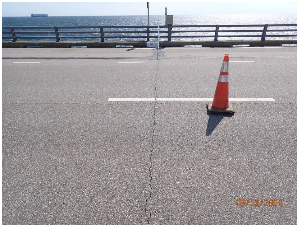
Photo 14: BNB167 – up to 1/8" wide transverse crack at expansion joint full width of roadway.
