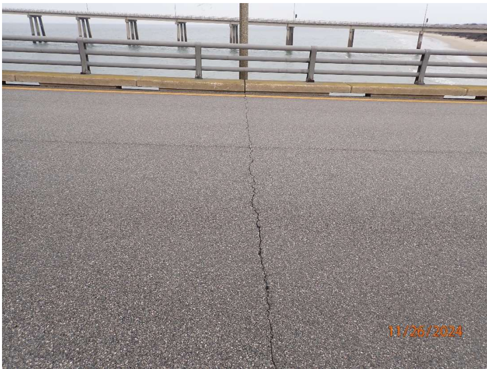
Photo 47: DNB2 Metal Bridge Railing & Expansion Joint - General Good Condition of Railing (Looking Northwest) and transverse crack over expansion joint.
