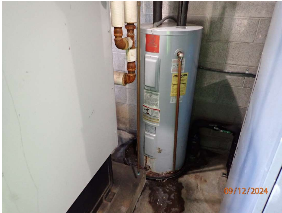
Photo 126 North Toll Plaza, Toll Office Building with water heater with minor leak.
