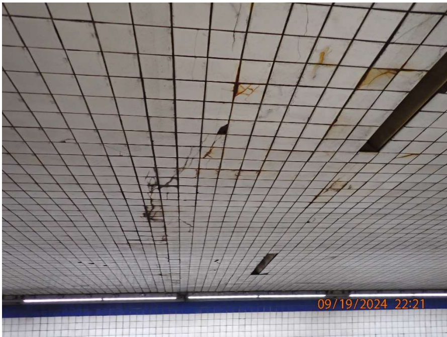
Photo 84: Tunnel Ceiling Slab – General View of Random Cracked Tiles in Tunnel Roadway Ceiling (Looking West)
