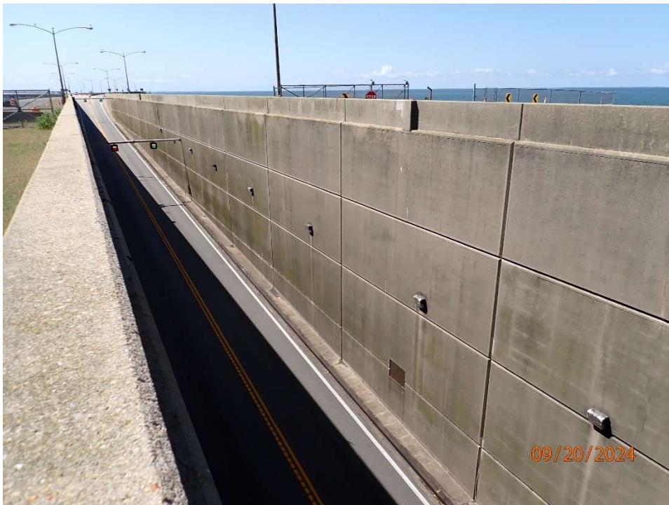
Photo 105: Portal Island 3 Open Approach Wall (west face); typical condition of approach wall.
