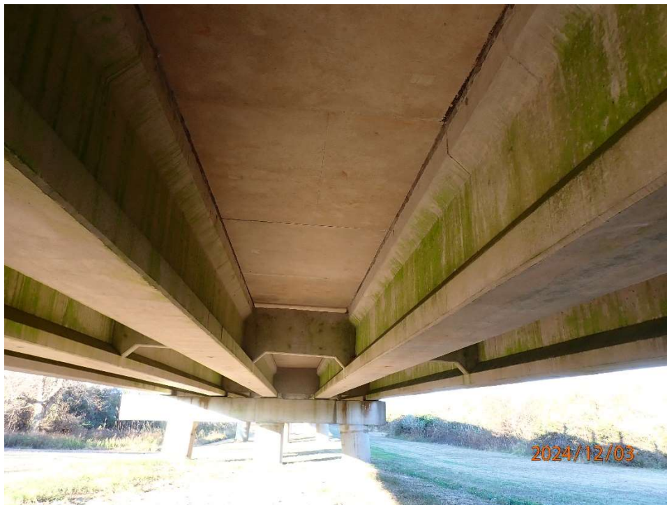
Photo 56 – DSB20 Superstructure in good condition. (Typical)
