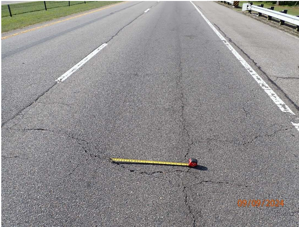
Photo 94: Approach Roadway (North); Asphalt with alligator cracking up to ¼" wide throughout.
