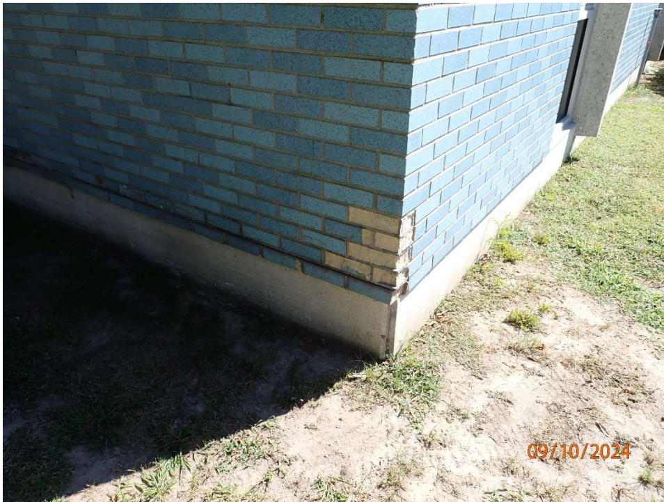
Photo 131: North Toll Plaza, Administration Building brick with minor deterioration at isolated locations. Overall, in good condition.
