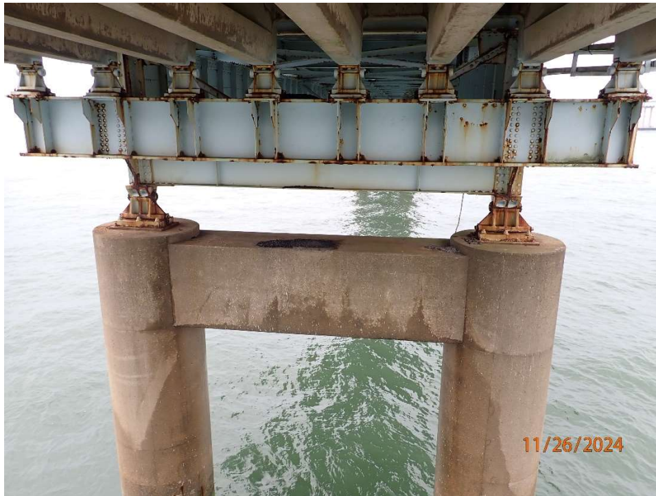
Photo 48: Superstructure – Typical condition of Superstructure with steel corrosion noted on up to 30% of surface area. Bearings in different degrees of expansion/contraction. Span 1 looking South.
