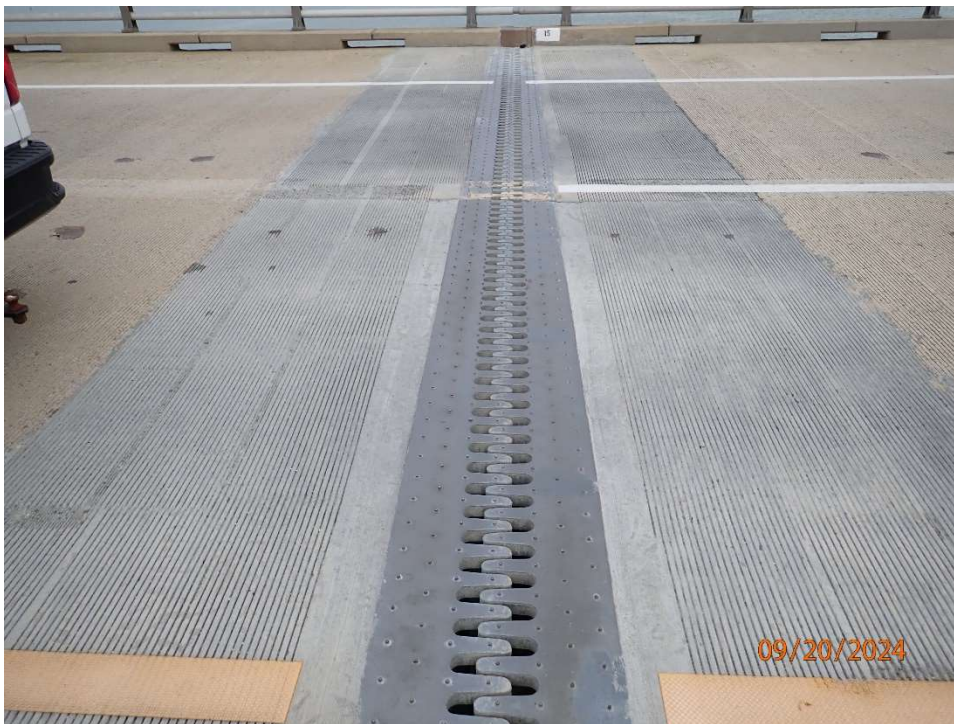
Photo 37: Modular Joint Seal – Typical Good Condition of Joint and Adjacent Deck Header, Pier 10 Shown (Looking West)
