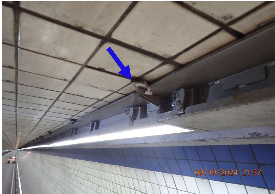
Photo 93: Tunnel Lighting Fixture – Loose anchorage/mounting hardware at East Station 469+60 (Blue Arrow) (similar at East Station 469+30)
