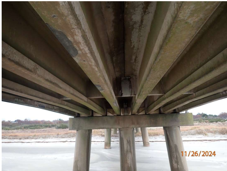
Photo 51: Superstructure & Substructure – Typical Good Condition of Beam and Piles (Span 5), Looking North.
