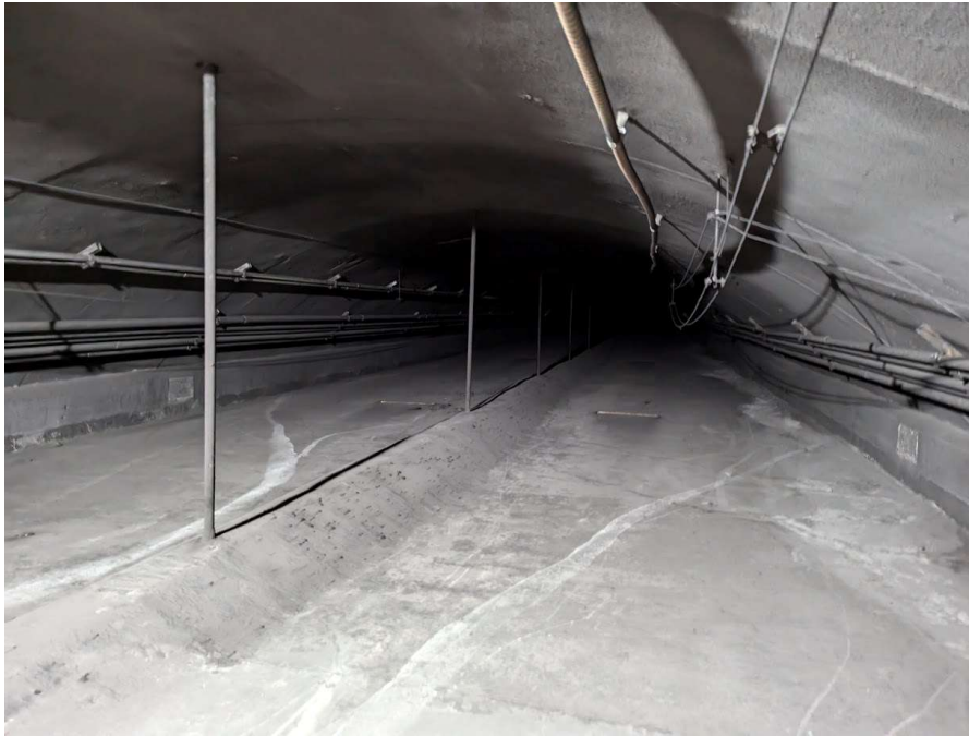
Photo 89: Exhaust Air Duct – General View along Tunnel Liner and Ceiling Slab (Looking North)
