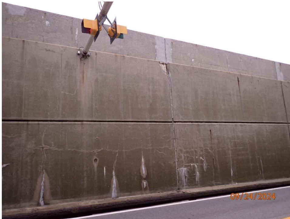
Photo 110: Portal Island 4; Open Approach Walls; hairline crack with rust staining and minor efflorescence.
