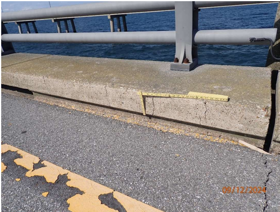
Photo 15: BNB165 – west curb with vertical cracks up to 1/8" wide.
