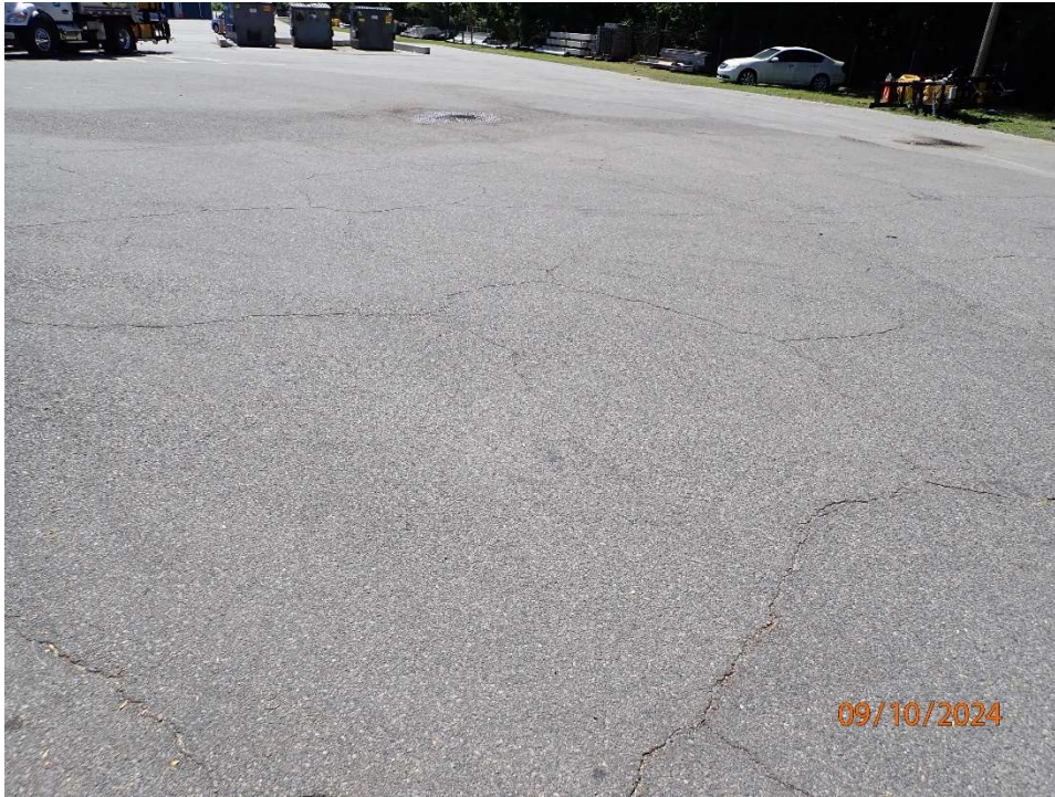
Photo 138: North Toll Plaza, Storage Yard and Parking in good condition with alligator cracking throughout up to ¼" wide. Isolated low areas with ponding water.
