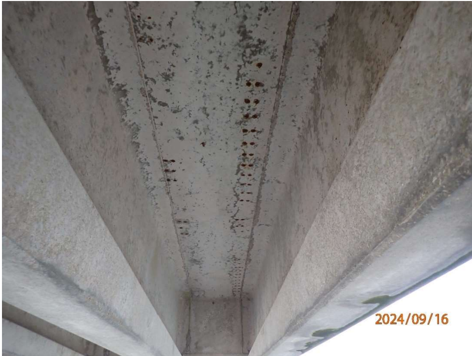
Photo 28: CNB197 Bay 7 typical underside of deck with exposed chairs at isolated areas.
