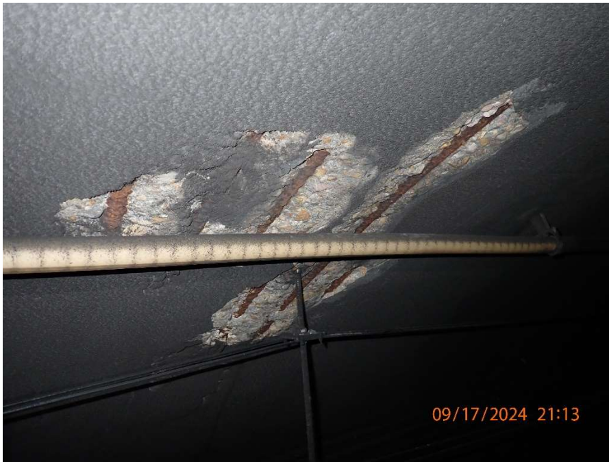
Photo 91: Exhaust Air Duct – General View of Random Spalling with Exposed and Corroded Reinforcement Steel in the Tunnel Liner (Looking West)
