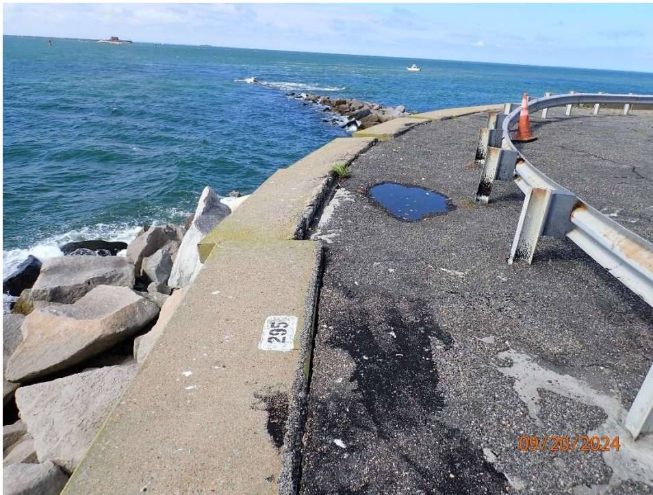
Photo 114: Portal Island 4 Splash Wall; Minor rotation to splash wall just south of sinkhole repair.
