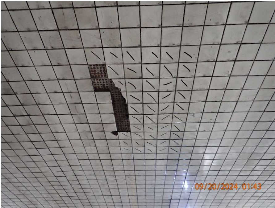
Photo 85: Tunnel Ceiling Slab – Isolated Area with More Significant Delaminated Concrete and Tile; and Missing Tiles in Tunnel Roadway Ceiling (Sta. 504+80 Looking South)
