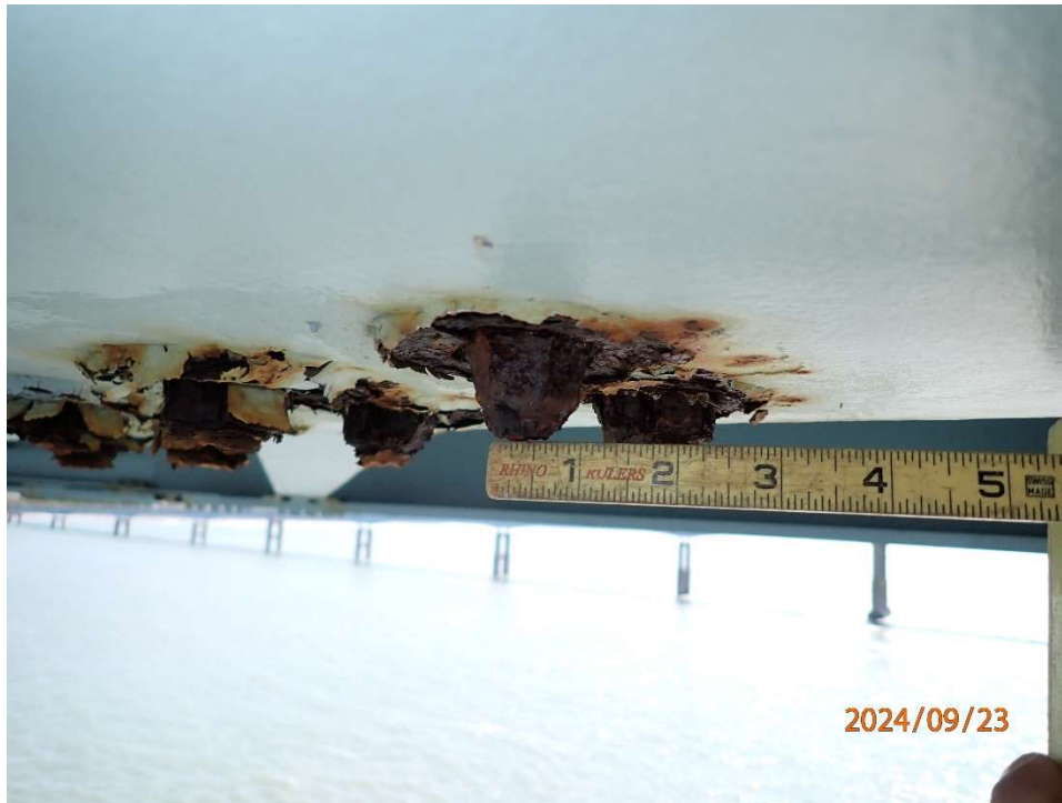
Photo 44 : NCB-SB – Typical Peeling Paint with Surface Corrosion and mushrooming of nuts on flange bolts.
