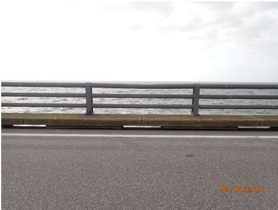
Photo 25: CNB201 Railing typically in good condition with minor impact damage at isolated locations.
