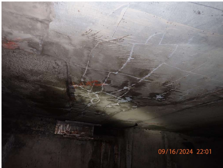
Photo 88: Fresh Air Duct – General View of Cracking with Efflorescence in the Invert Slab (Looking East)
