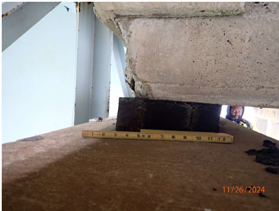
Photo 64: FIBNB4 G4 beam end spall 5" L x 8" H with up to 5% section loss on bearing area.
