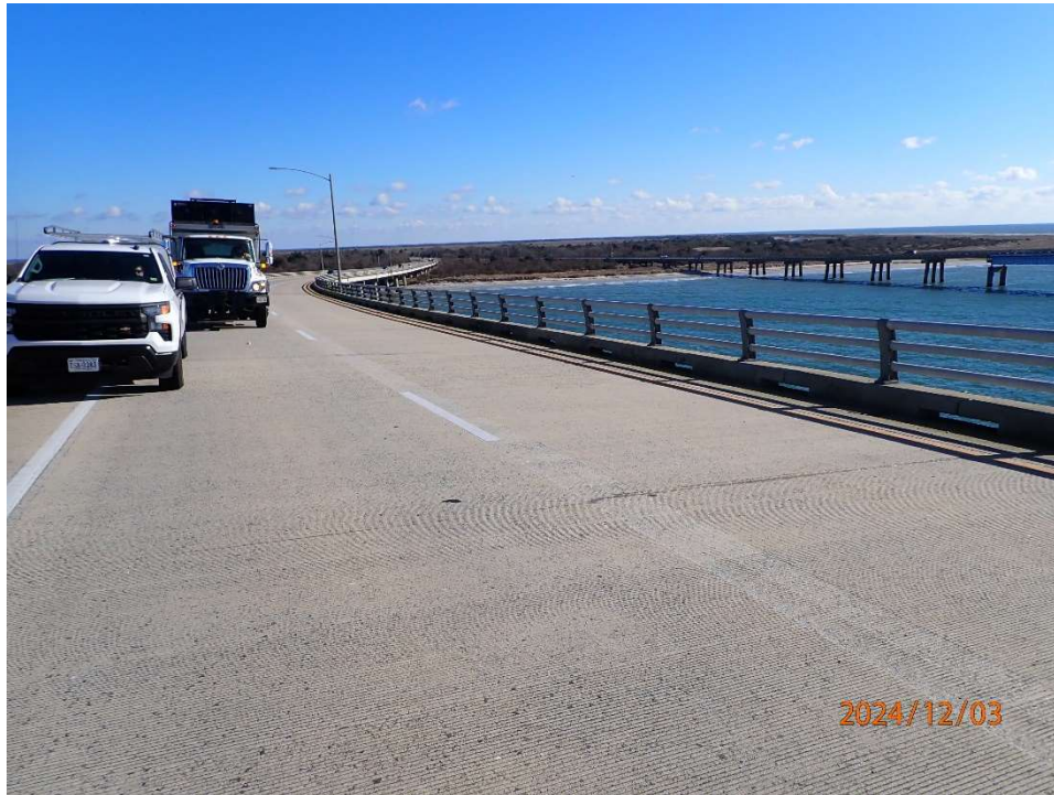
Photo 55 – DSB2 Deck in good condition with up to 1/16" wide cracking at isolated locations.
