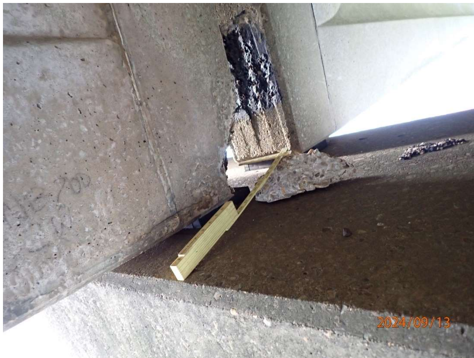
Photo 20: BNB200 at Beam 2 on Bay 2 side, beam end delamination/spall 18" L x 1' H x 6" back x 2" deep with exposed reinforcement with up to 50% loss of section at beam end and partial bearing loss.
