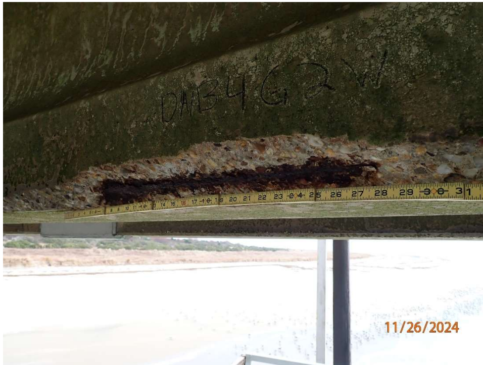
Photo 50: DNB-4 G2, Beam 2 Bay midspan 3' long x 6" high x 4" under with 1 exposed prestressing strand (L1) up to 50% section loss.
