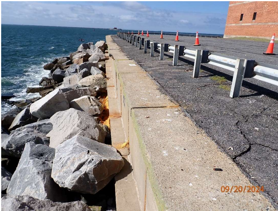
Photo 112: Portal Island 4 Splash Wall; Repair to previous sinkhole with urethane material out of joints.
