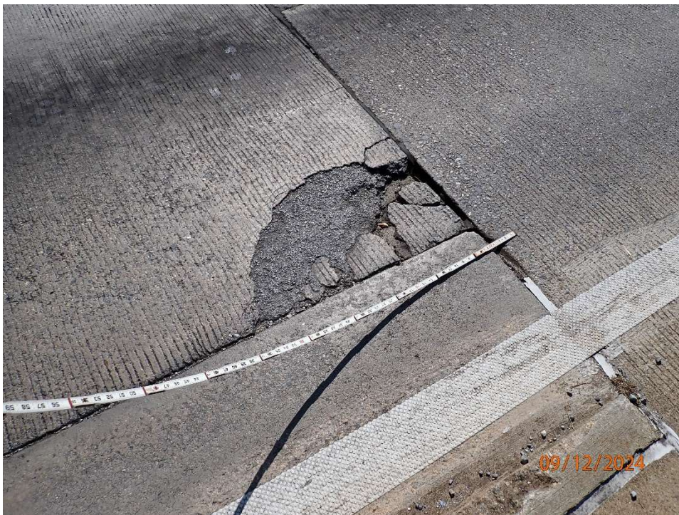
Photo 129: North Toll Plaza, Toll Booth and Canopy, isolated pothole 18" diameter x 2" deep.
