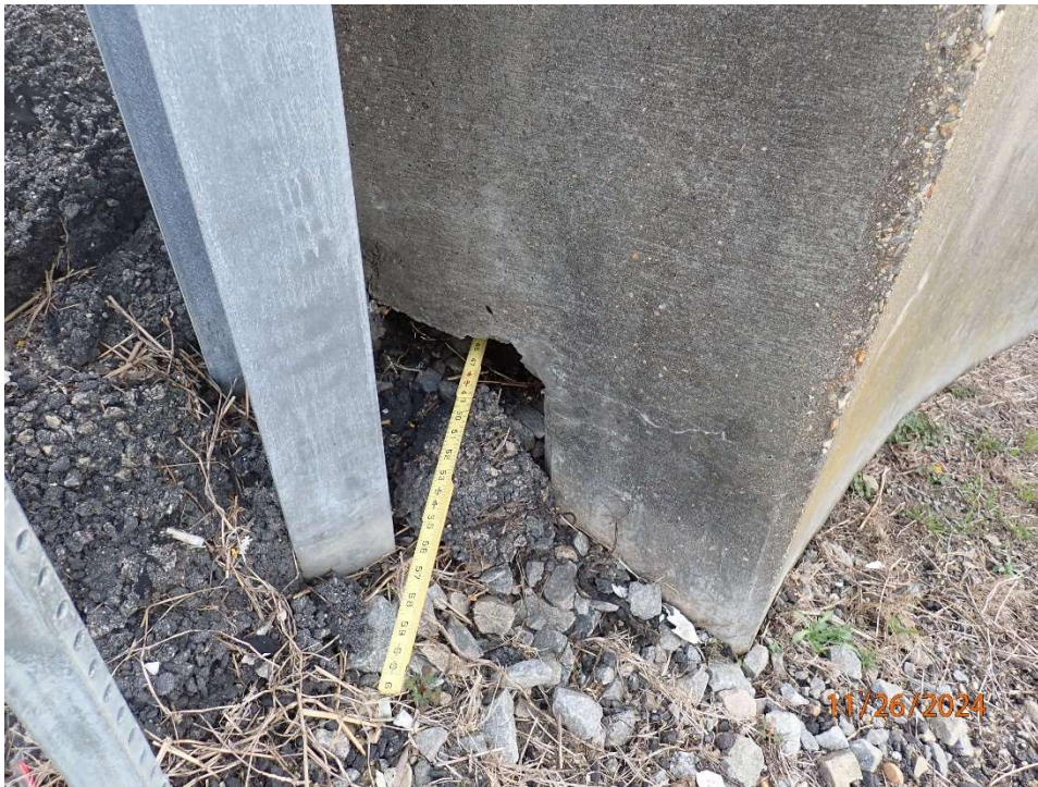
Photo 54: West wingwall undermining up to 1' wide x 6" high x 4' under.
