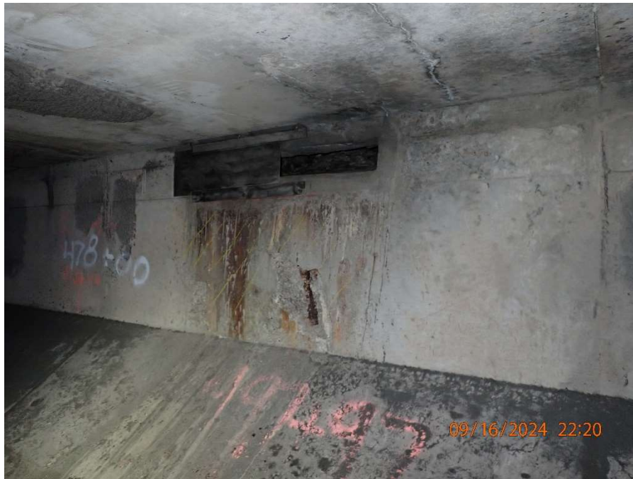
Photo 87: Fresh Air Duct – General View of Delamination and Spalling in the Tunnel Liner (Looking East)
