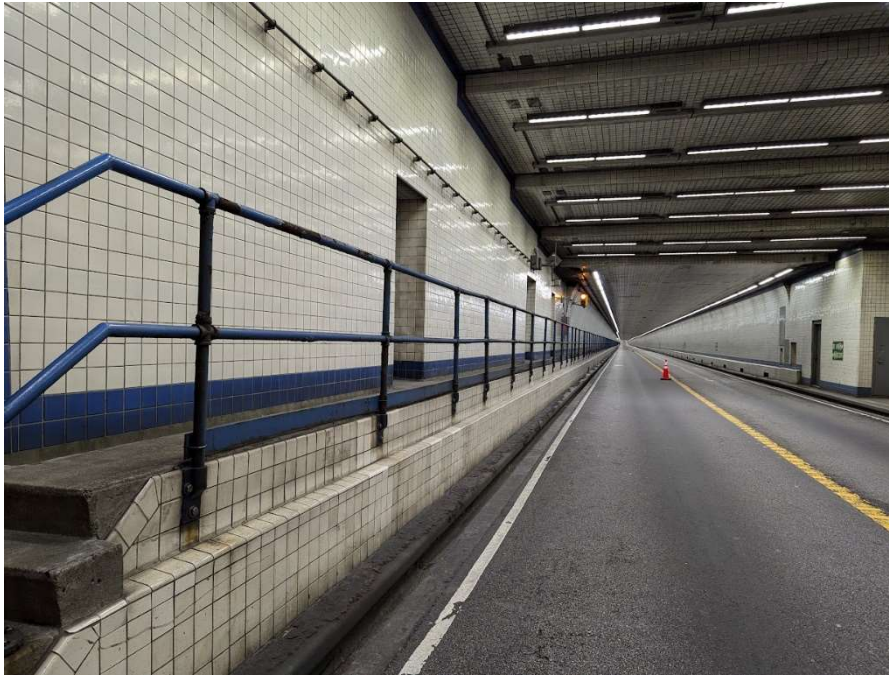
Photo 83: Tunnel Roadway – General View of the Concrete Barrier (Lined with Tile), Curb, Sidewalk, Pedestrian Railing, and Tunnel Liner Wall (Looking North)
