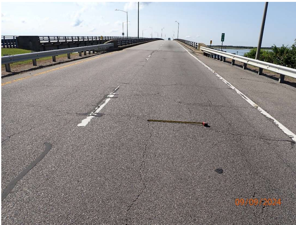
Photo 95: Approach Roadway (North) near FIB Bridge; Asphalt with alligator cracking up to ¼" wide throughout.
