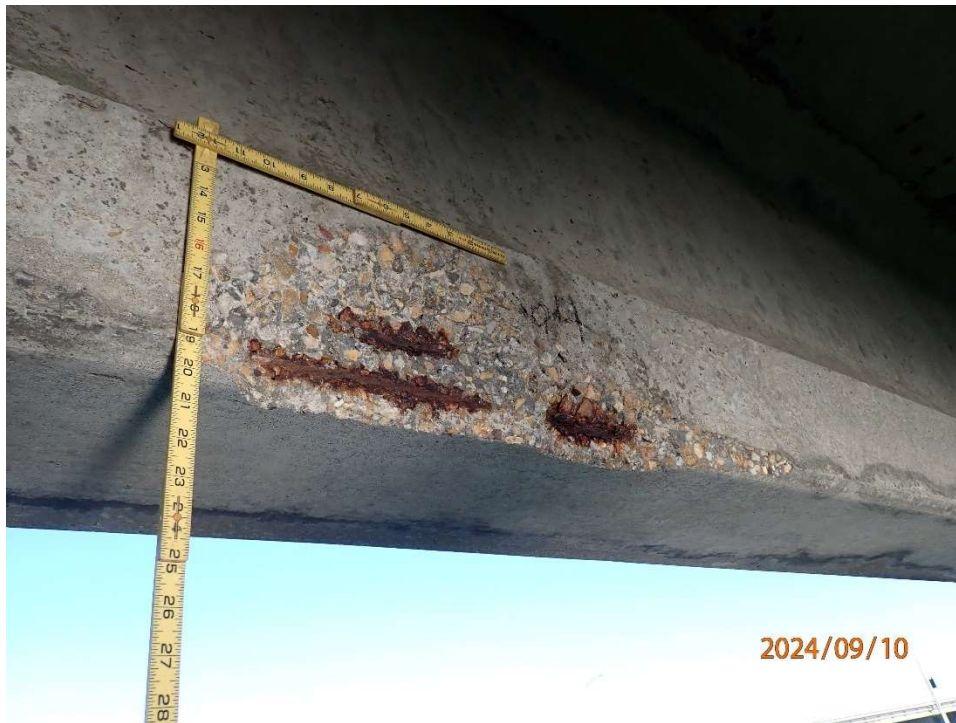
Photo 8: ANB204.5 – Beam 8, Bay 7 at 1/3 span spall 30" L x 8" H x 1" D with 2 exposed prestressing strands (L1 and L2) with up to 20% section loss.
