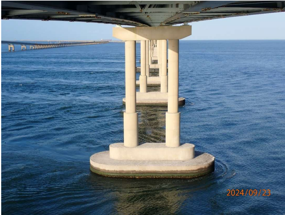
Photo 40: Substructure – General Condition of Pier Substructure
