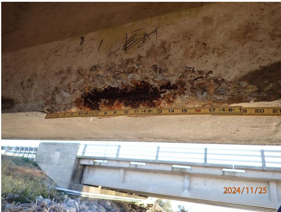
Photo 74: FSB8 Beam 1, Bay 1 spall 18" L x 5" H x 2" under x 2" deep with 1 exposed prestressing strand with up to 10% section loss.
