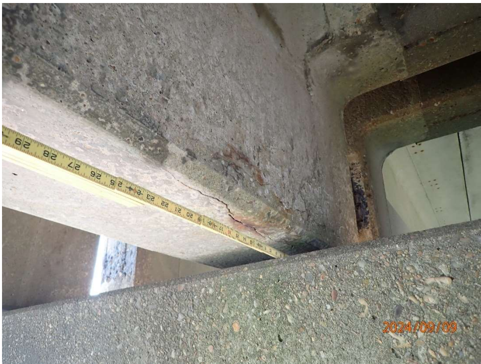
Photo 6: ANB182 – Beam 2 at Bent 183: 2' long 1/8" wide crack on underside of beam.
