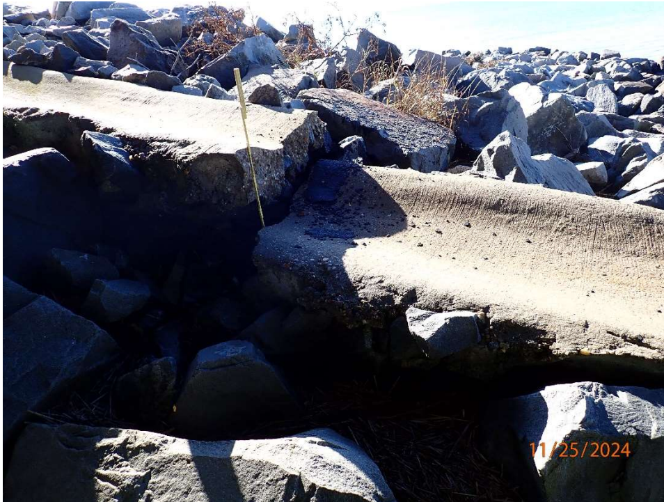
Photo 70: Abutment – drainage swale on west end settled and disconnected.
