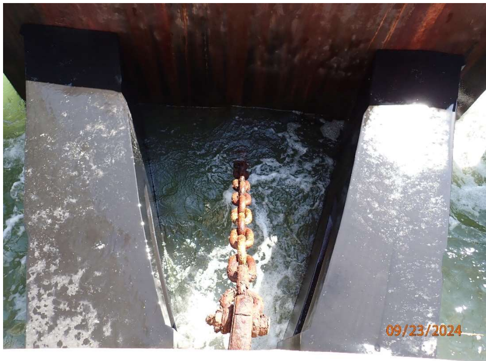
Photo 45: Fender System – Typical Minor Corrosion of Chain between Pier 9 Footing and Fender System (Looking South)
