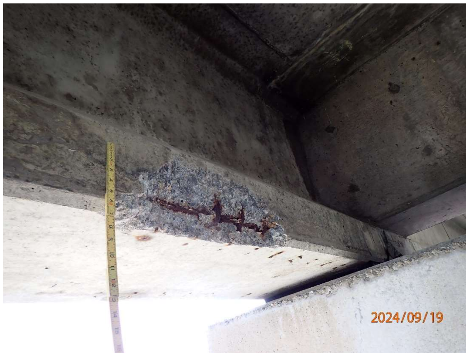
Photo 35: CSB90 Prestressed Girder 1 spall with exposed prestressing (L1) and reinforcement. Spall measures 2' L x 7" H x 2" under x 1-1/2" deep with 20% section loss to prestressing strand and reinforcement.
