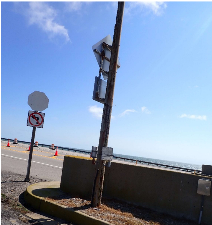
Photo 117: Portal Island 4 Concrete Light Pole; typical condition of poles with areas of spalls with exposed reinforcement up to 20% section loss of reinforcement.
