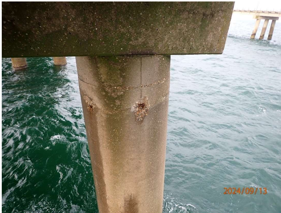
Photo 17: BNB199 – Pile A; 12" H x 6" W x 1" Deep spall with exposed reinforcement with up to 10% section loss.
