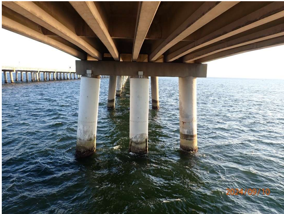
Photo 9: ANB202 – Substructure with fiberglass jackets . Jackets typically in good condition with isolated areas of jacket failure at waterline.
