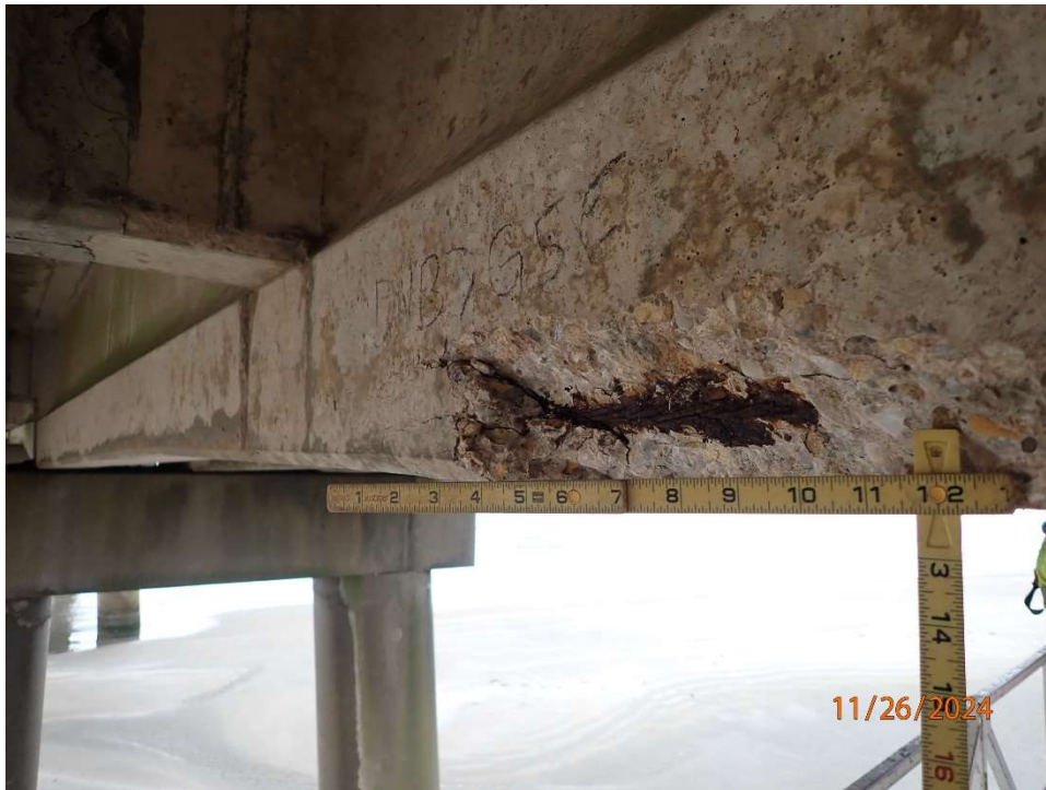
Photo 53: Prestressed Concrete Girders, DNB-7 G5, Beam 5 midspan 3' long x 5" high x 5" under x 2" deep with 1 exposed prestressing strand up to 100% section loss.
