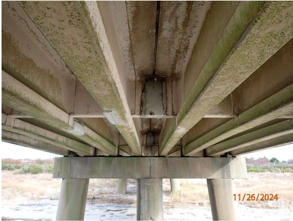
Photo 52: Typical Good Repair Patch on bottom of girder in Span 6 in 2 locations. Looking North.
