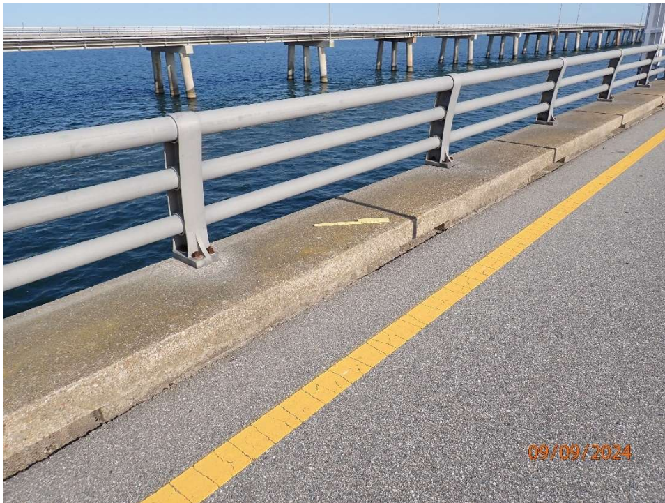
Photo 2: ANB181 Metal Bridge Railing – Typical good condition of bridge railing and curb.
