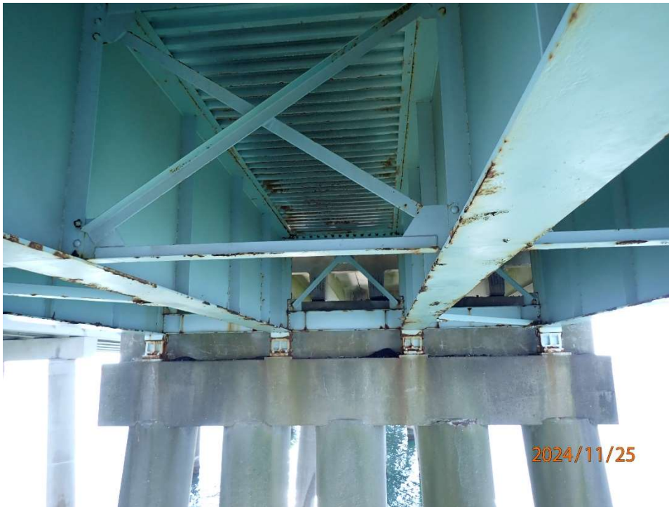
Photo 73: FIBSB Superstructure in good condition with isolated corrosion noted on bottom flange.
