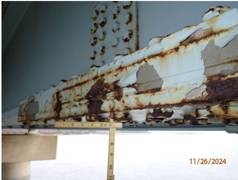
Photo 65: FINB1 Steel Superstructure at splice plate with blistering paint with surface corrosion.
