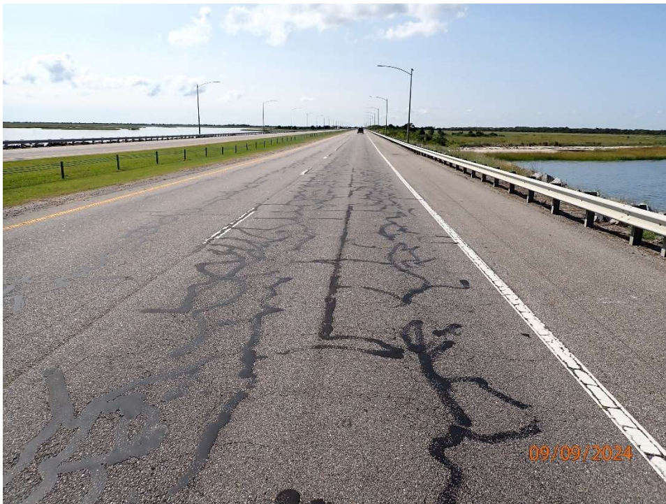
Photo 99: FIB Causeway looking south; Asphalt with up to 1/8" alligator cracking with majority sealed.
