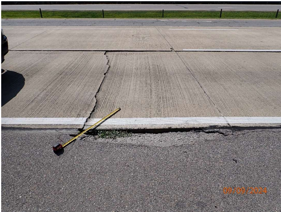
Photo 97: Approach Roadway (South) headed north approx. 675' south of gate; pothole and concrete pavement settled up to 1" with up to ¼" wide transverse crack.
