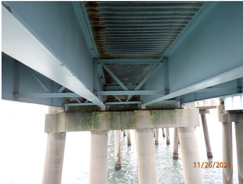
Photo 63: FIBNB1 Superstructure in good condition with isolated coating loss and surface corrosion.
