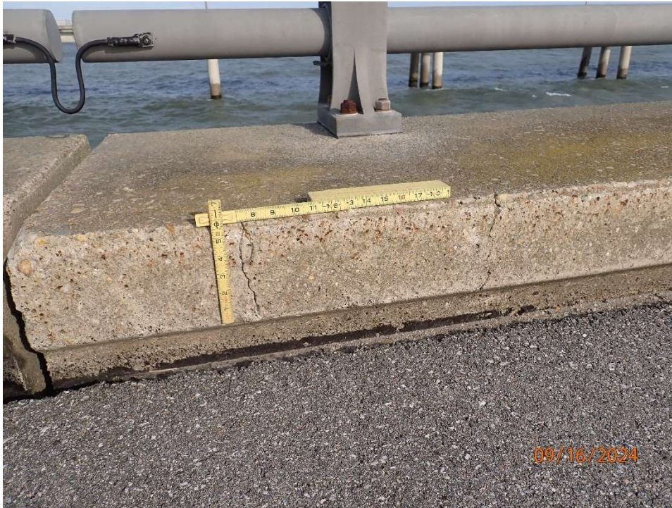
Photo 26: CNB203 Curb typically in good condition with minor cracking noted on face of curb at isolated locations.
