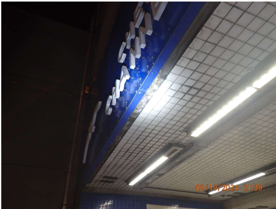
Photo 80: Tunnel Portal – General View of the Island 3 Portal Spalling (Looking West)
