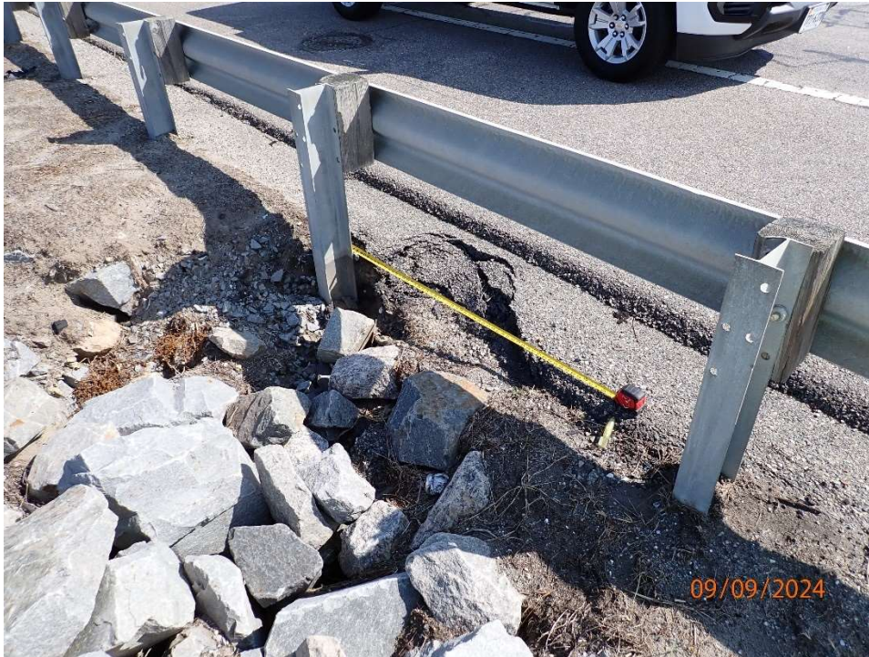
Photo 100: FIB Causeway headed south; Pothole/sinkhole at shoulder/guardrail with riprap. Sinkhole measures 42" wide x 24" long x 3" deep.
