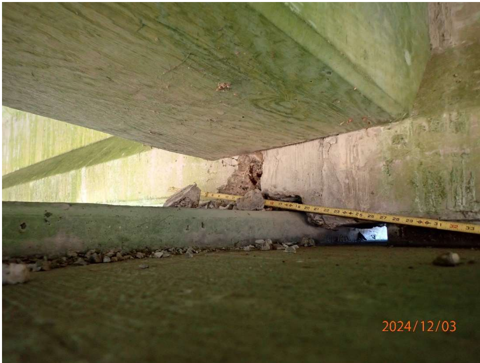
Photo 58: DSB20 Bent 20 Beam 5 Bay 4 with beam end spall; spall up to 6" H x 6" L x 4" Deep with exposed reinforcement. Spalls noted at isolated locations.
