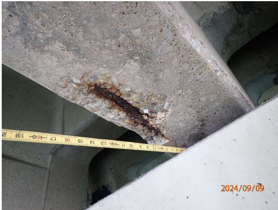
Photo 7: ANB191 – Bent 192 at Bent 5, Bay 5 spall/delam 25" L x 2" H x 8" under x 1" deep with exposed reinforcement with up to 20% section loss.
