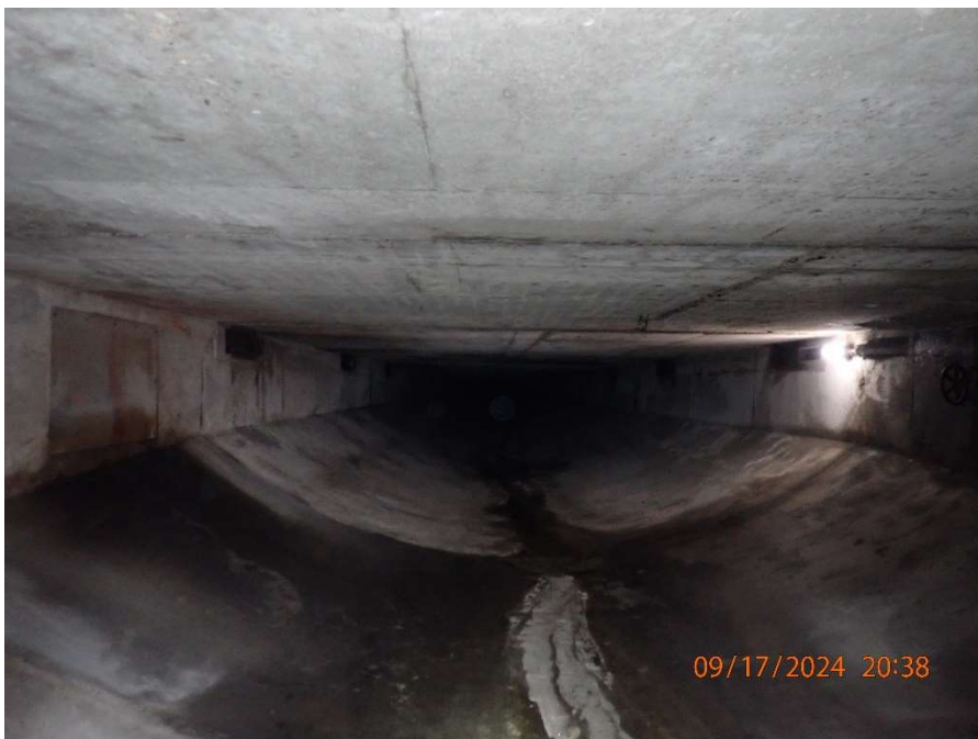
Photo 86: Fresh Air Duct – General View along Tunnel Liner and Invert (Looking North)
