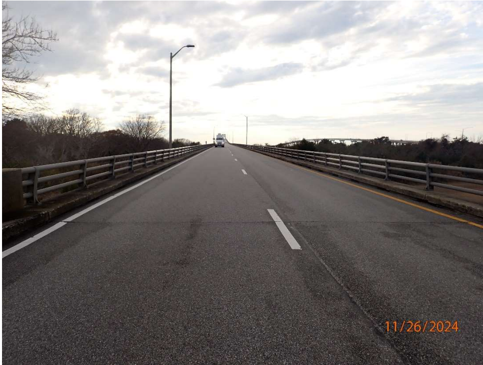
Photo 46: DNB Wearing Surface - General Good Condition of Deck and Wearing Surface (Looking South)
