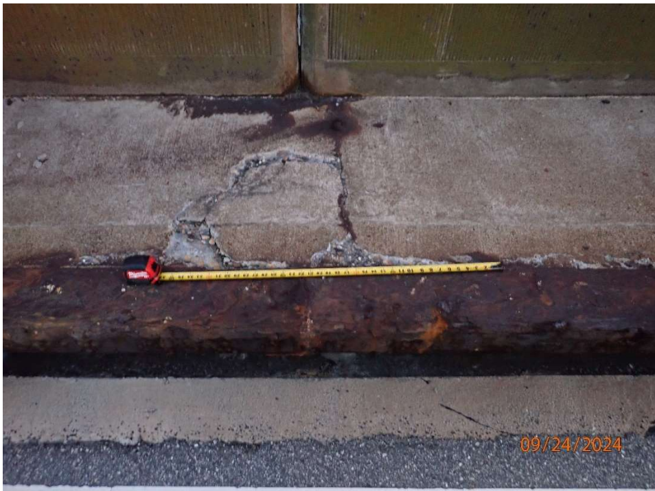
Photo 103: Portal Island 3 Approach Roadway; corrosion to rub rail throughout with isolated delaminations to sidewalk/curb.
