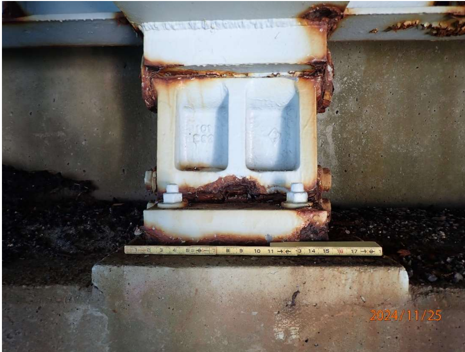
Photo 75: FIBSB3 Bearings have pack rust up to ¼" thick typical for bearings.
