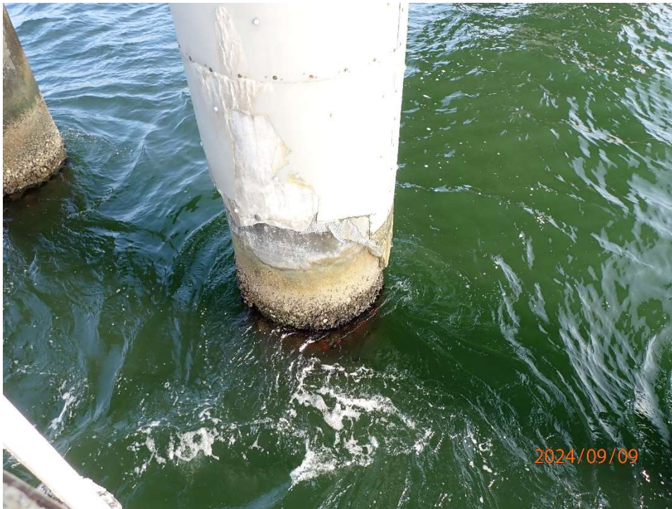
Photo 5: ANB181 – Pile B – Jacket missing full circumference bottom 8' with missing grout.
