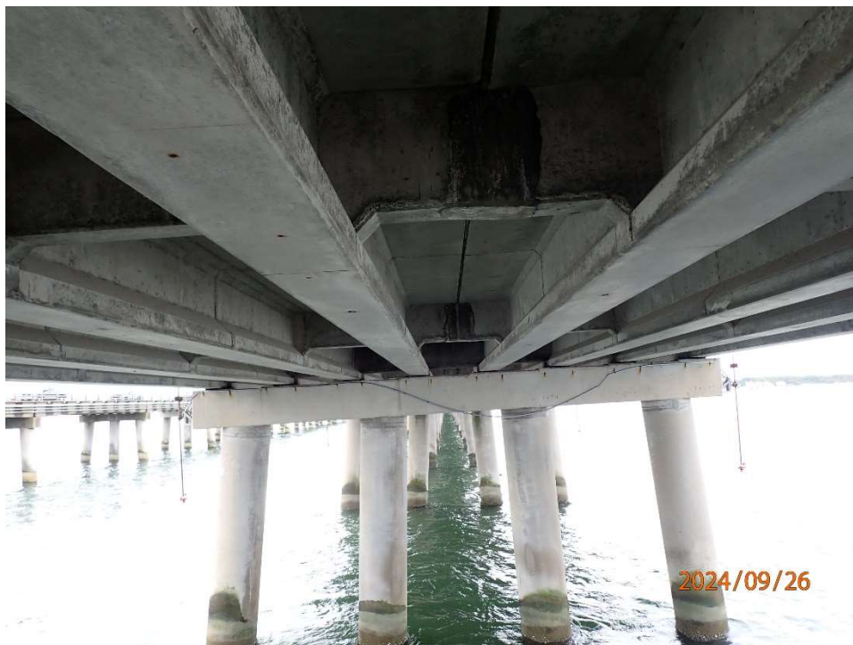
Photo 11: ASB71 Bent 71 north face typical good condition. Bent 71 has detached conduit for navigation light at bent cap.
